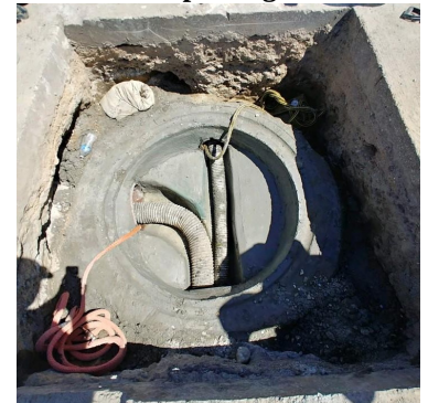
Gravity Bypass - Manhole
